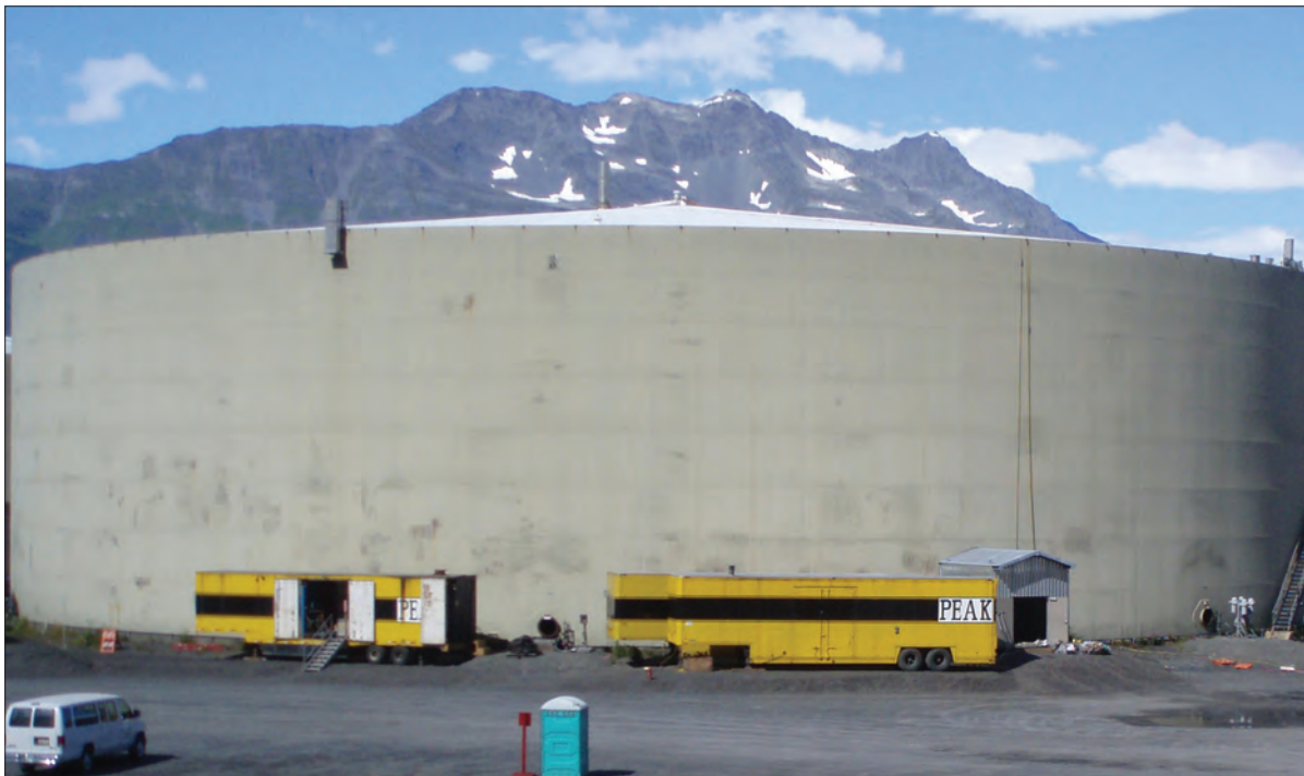
Below: Exterior of the tank inspected in 2004. An entry hole like the one above can be seen in the photo below between the yellow trailers. Photos by Tom Kuckertz.
