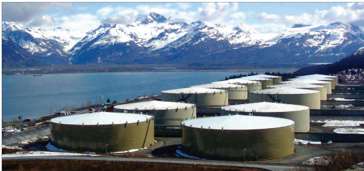
The terminal's storage tanks hold crude oil from the trans-Alaska pipeline until it can be loaded onto tankers. Photo by Linda Robinson.
