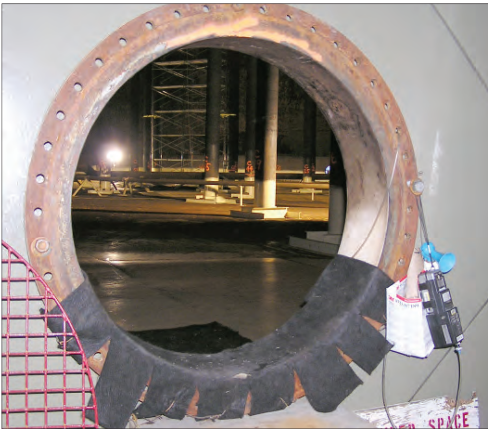
Above: The interior of one of the tanks after a 2004 inspection and cleaning.
